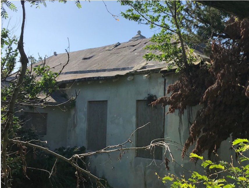
The roof on Dubloon Cottage looks unrepairable
