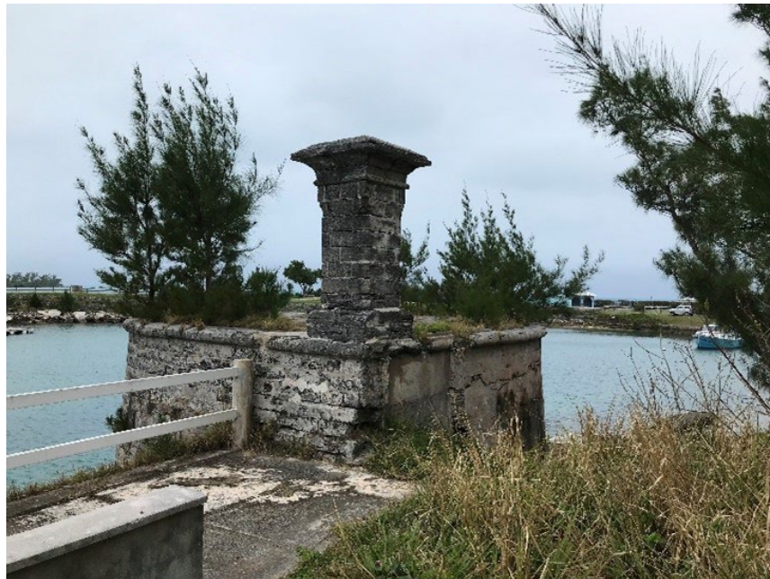
Figure 4: The bathhouse turned cookhouse is in danger of being taken over by the fast-growing casuarina.
