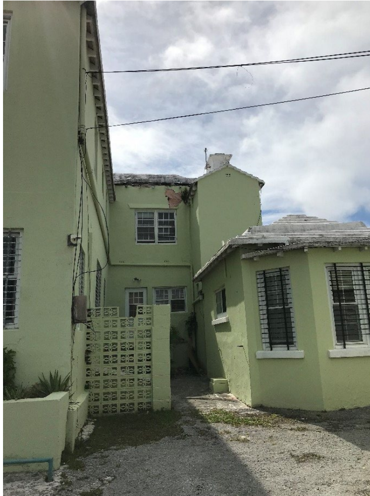
The side entrance to Archlyn Villa is not a pretty sight. Are the window bars really necessary?
