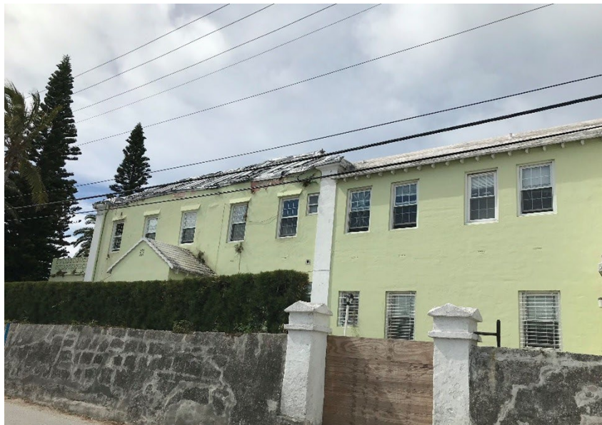
The roof on the original section of Archlyn Villa appears to have had hurricane damage.
