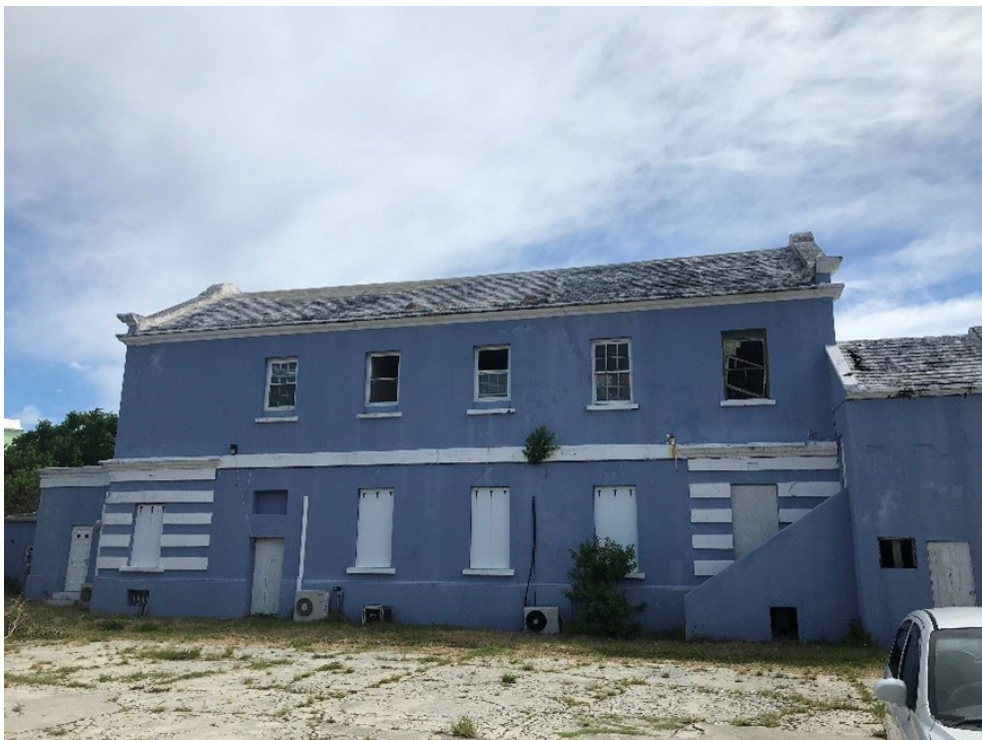
The east side of Victoria and Albert Lodge in 2022. With some community involvement and government support the damage could be repaired.
