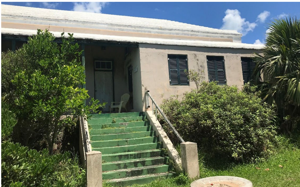
Now called Nonsuch House, this is the front view of the West Hospital Ward. A portion of the verandah was enclosed many years ago. The eastern wing of the building in particular is now in very poor condition.
