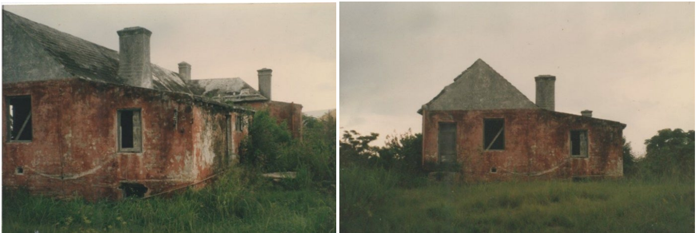
By 1999 the condition of the Ratteray Homestead had further deteriorated but could still have been saved from total ruin.
