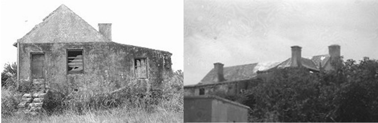
The roof of the Ratteray Homestead was still intact in 1991 and the building could still be repaired.
