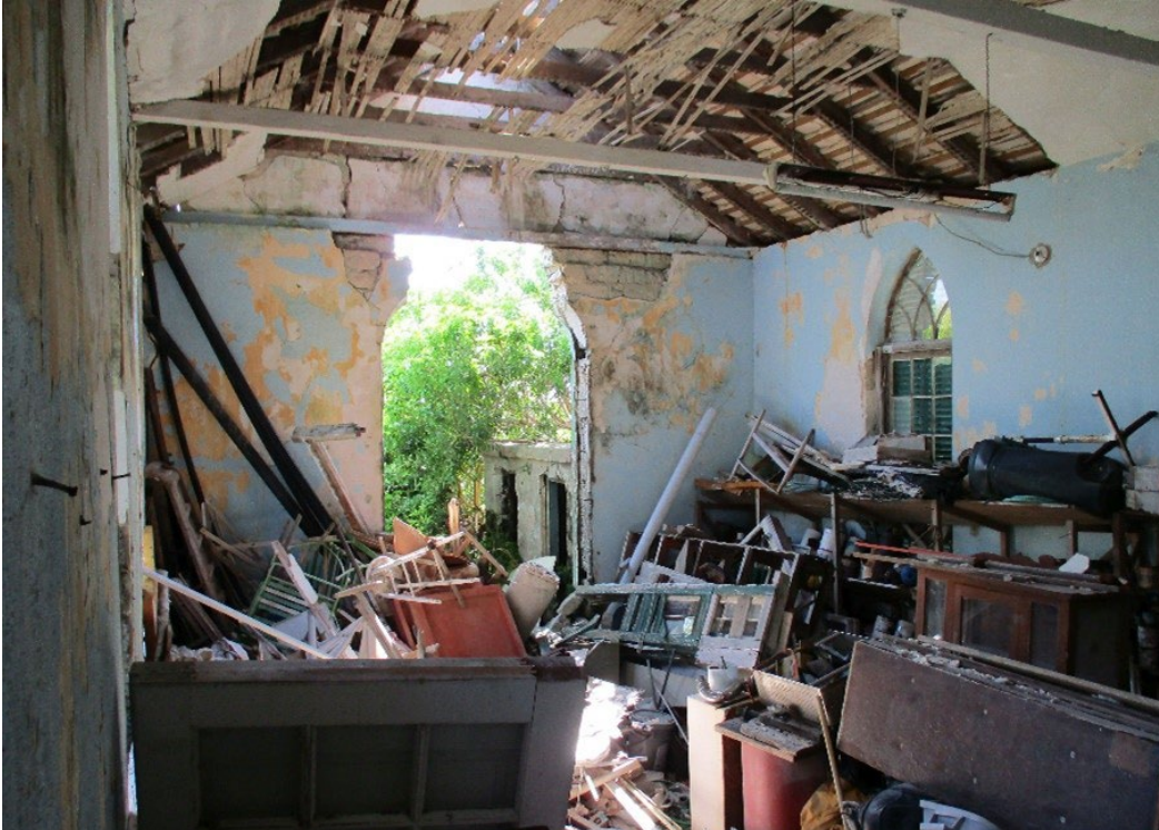
An interior view shows that the last tenant did not even remove his materials. The ruined toilets show through the open door.
