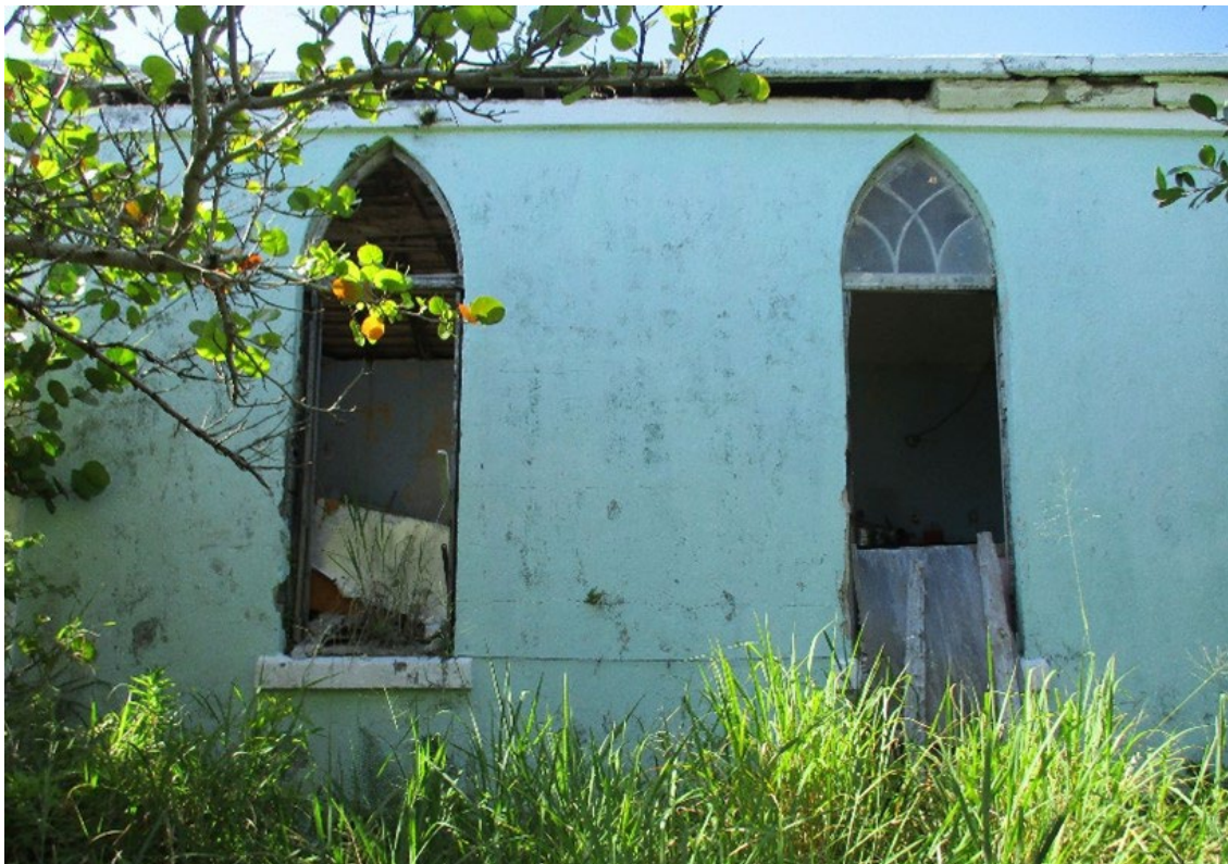
The south side of the building has suffered hurricane damage.
