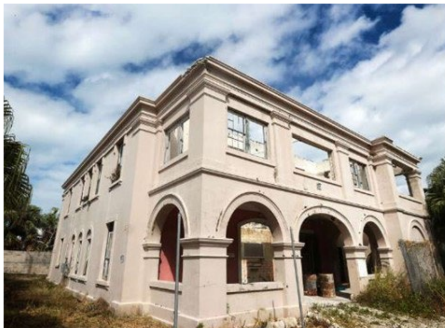
Teucer House suffered extensive damage from fire in October 2013.
