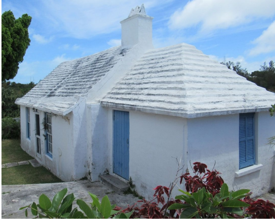
The roof of Montpelier Cottage is riddled with cracks and vegetation is growing through the windows.
