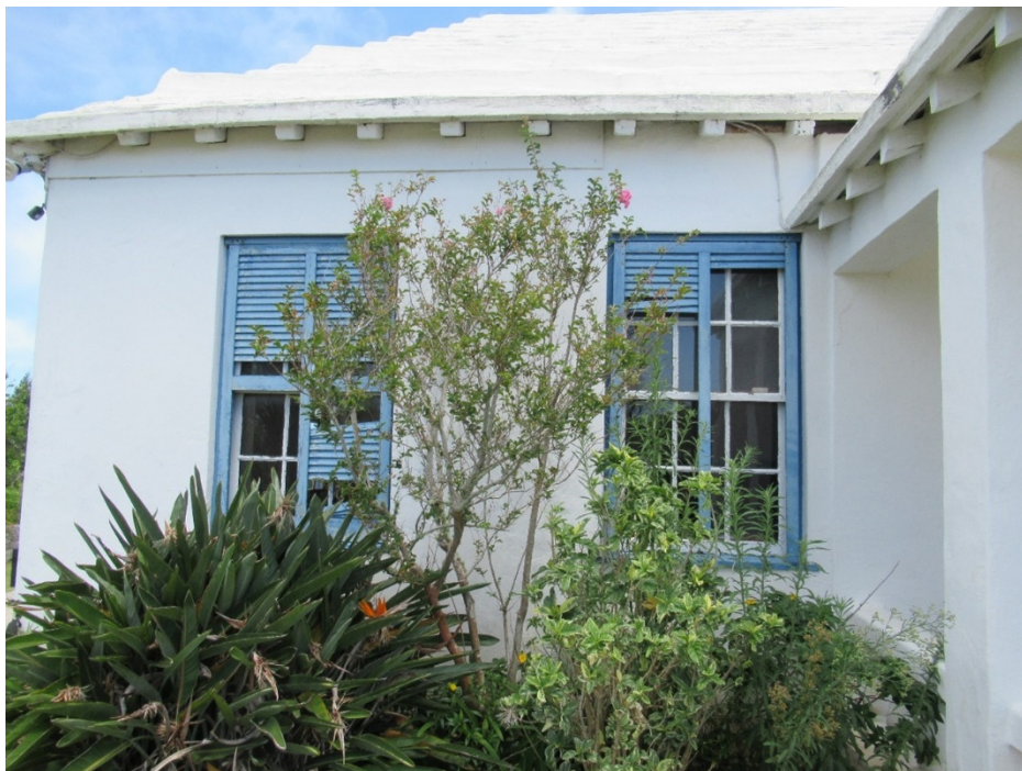
Montpelier's shutters have been allowed to fall to pieces.
