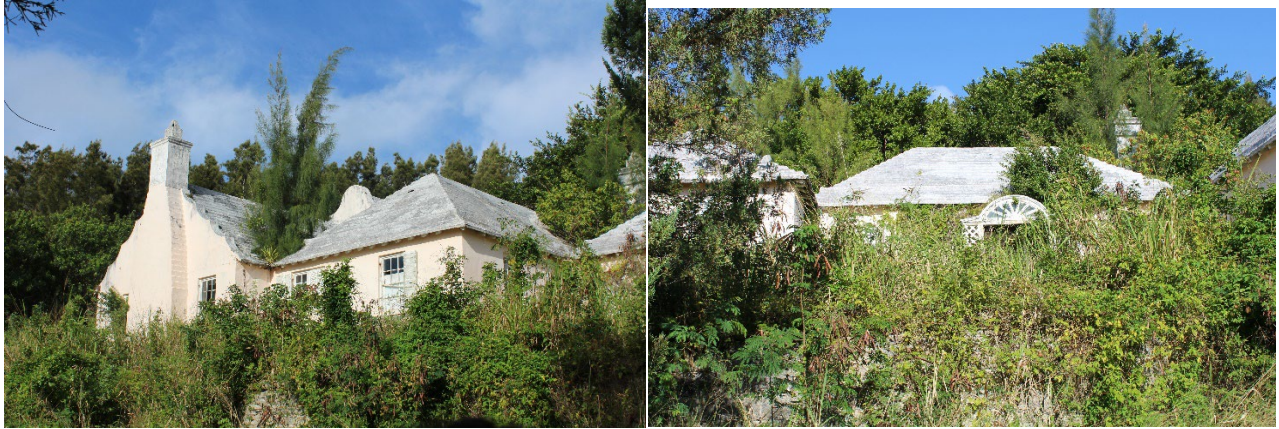
By 2019 Southlands was being taken over by invasives. Note the casuarina growing out of the roof.
