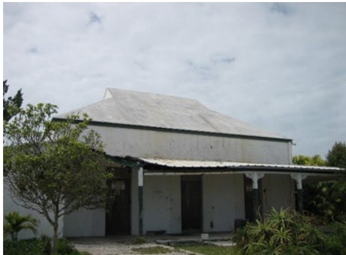
The ballroom's gambrel roof was still intact in 2006 as were many of A.D. Hollis' wooden brackets.
